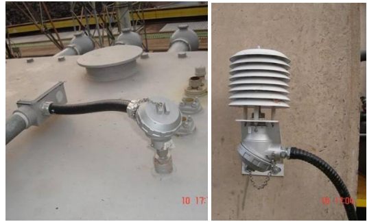
Fig. 6. Top oil temperature (left) and ambient temperature sensors.
