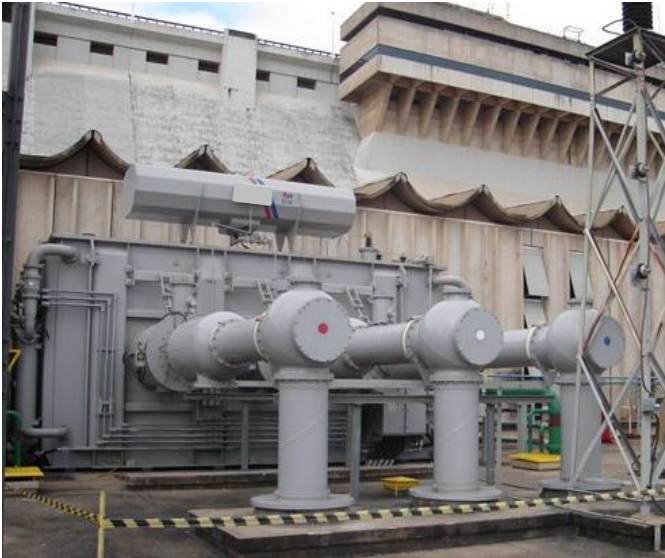
Fig. 3. One of the step up transformers, 378 MVA 13.8/550 kV.
