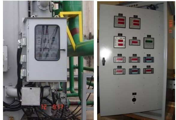
Fig. 8. Intelligent Sensor Panel (IEDs) on a transformer's body.
