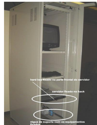
Fig. 9. Control Room monitoring Server.
