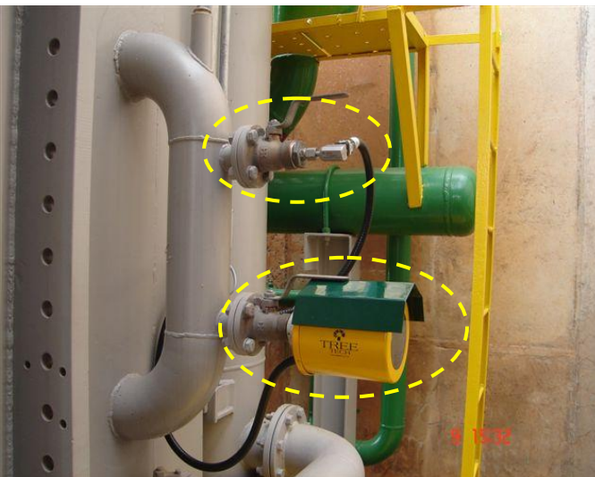
Fig. 5. Moisture monitor (above) and gas in oil monitor.
