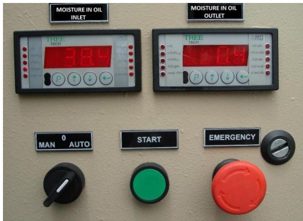
Fig. 2. View of the drying-out system data-monitoring sensors and control panel
