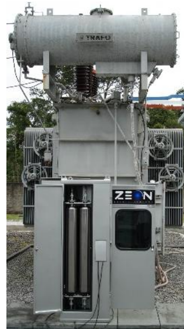
Fig. 1. Drying-out system installed on an in-service power transformer
