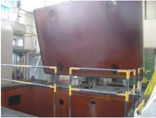
Fig. 8. Thermo chamber for drying-out processes.
