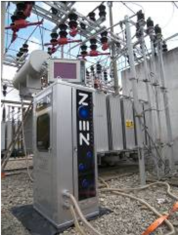
Fig. 12. Drying-out system installed on an in-service power transformer (12MVA).
