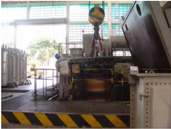
Fig. 9. Vacuum chamber for drying-out processes.
