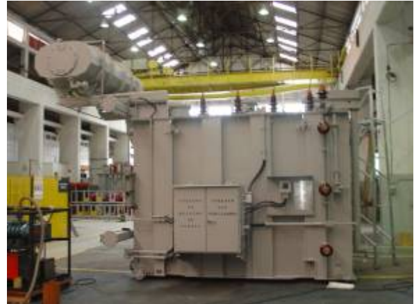
Fig. 6. Transformer used for PDC measurements and traditional drying-out.
