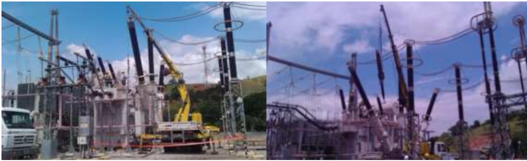
Figure 07: Cemig's crew replacing the defective bushing.
