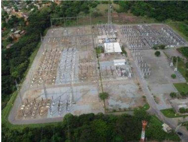
Figure 02: Aerial view of Cemig's Mesquita Substation, located in the eastern Minas Gerais region.
