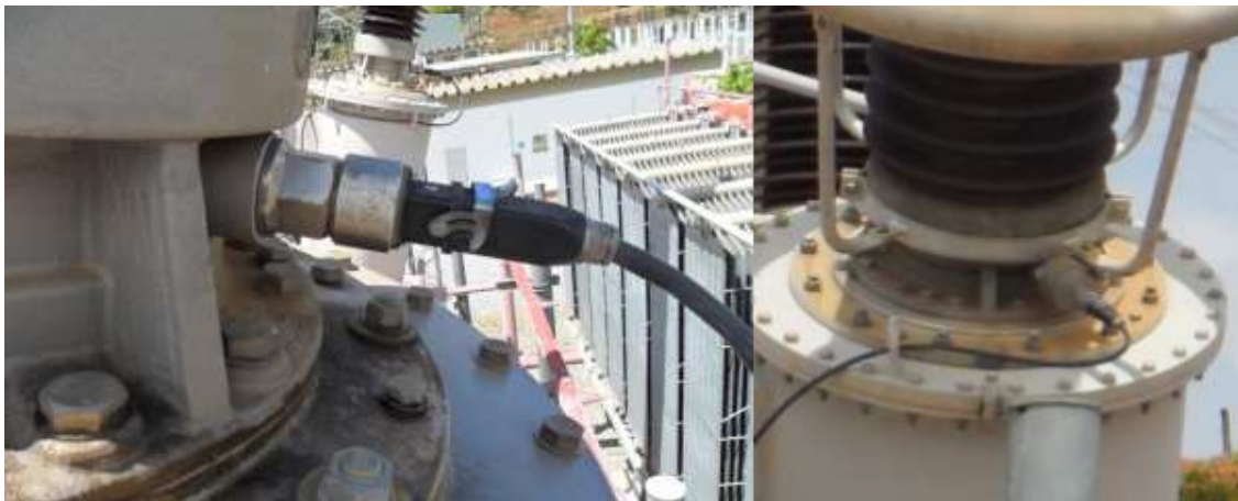
Figure 04: Detail of the tap adapters used in the BM bushing monitoring system installed at Mesquita Substation.
